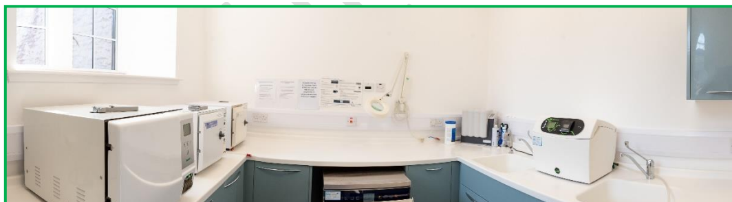
Figure 2.1 A dedicated decontamination unit
